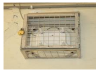
Wi-Fi access point
