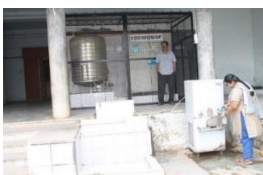
RO water plant
