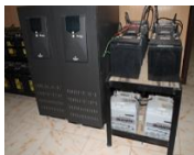
UPS back up
